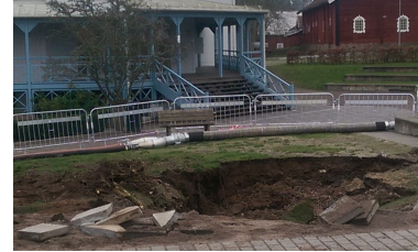
Picture of sink hole by Ogar93 via Wikimedia Commons
